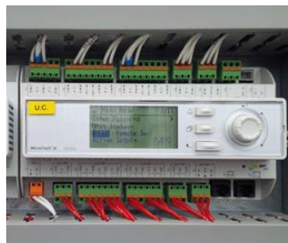
Controller box upgrade
